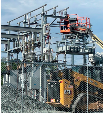
The collector substation for Bear Branch Solar is nearing completion with energization planned for August.
