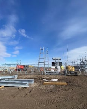
Construction of the Goldeye 620S Substation located on RR 151 is approximately 45% complete.
