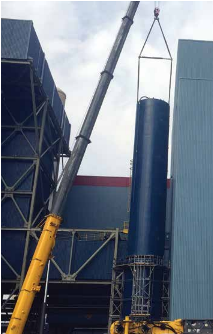
Contained within a 105' silo, the newly installed DSI system injects hydrated lime into G3's flue gas stream to further reduce SO 2 emissions from G3.
