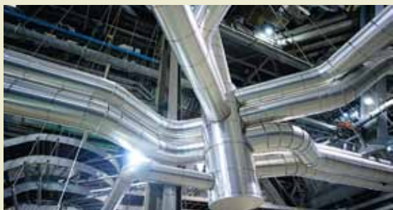
Steel piping network inside Keephills 3.
